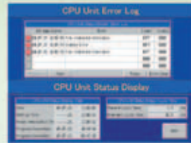
PLC CPU Unit monitoring screen
